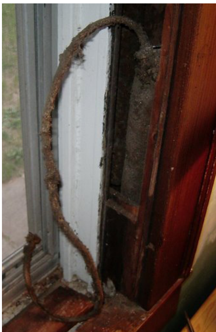
Broken Sash Cord and Weight
