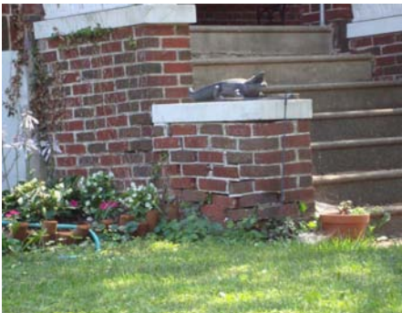
Brick Piers with Missing Mortar
