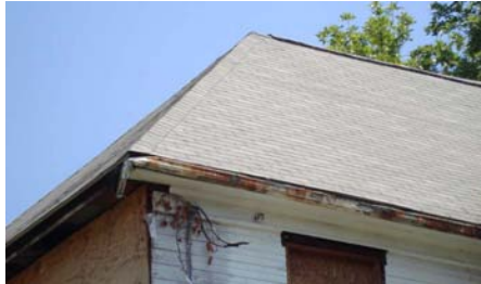
Gutters in poor repair can overflow and increase moisture levels in the soil around foundations.
