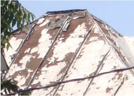
Metal Roof in Poor Condition
