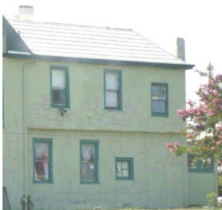
Poorly Patched Cracks on a Stucco Home
