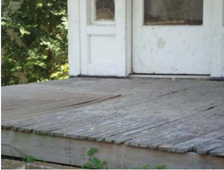
Sagging Porch Floor
